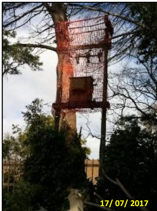
Figure 14: The enclosed transformer box at Veels-Te-Ver.
